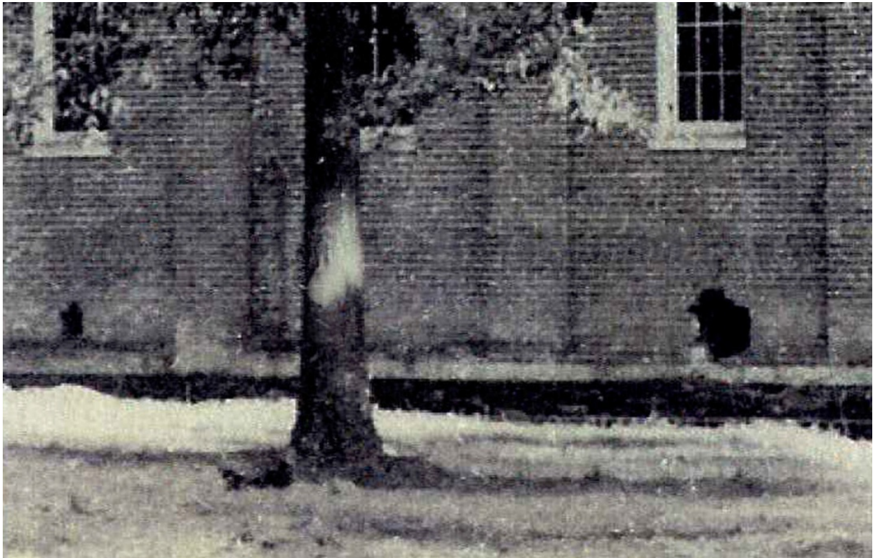
Close up picture of holes in wall - Picture is blurred because of magnification
